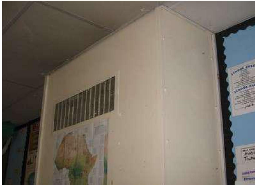
Warm Air Cabinet Heating. Classroom Cwmcarn School.2009
