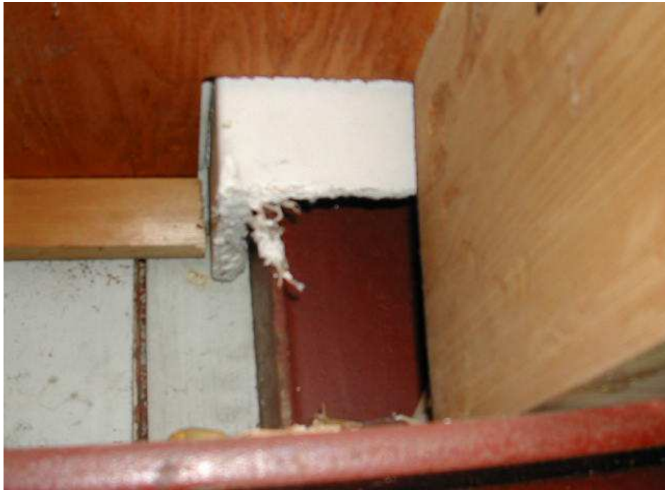
Plate 5: Exposed badly damaged asbestos cladding
